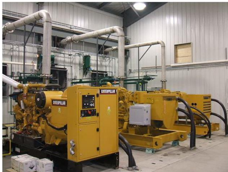
Figure 1: St. Lewis – Diesel Generators in Power House
