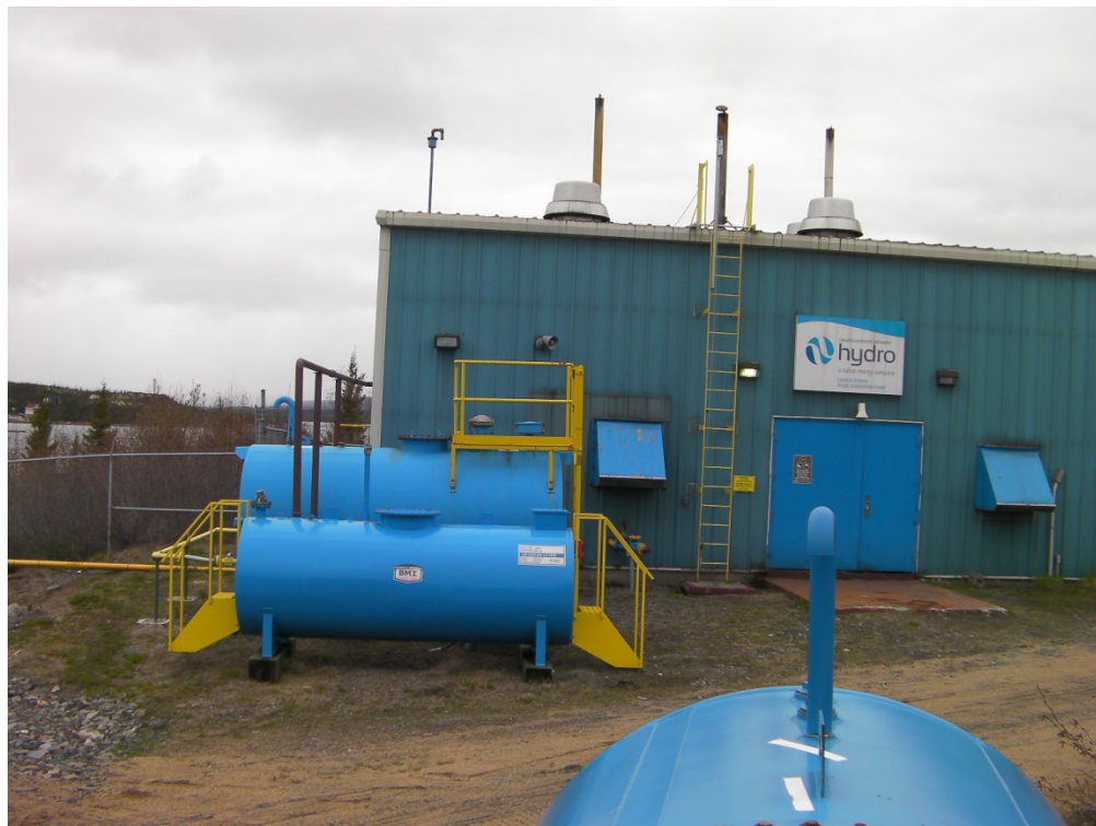
Figure 4: Charlottetown Generating Plant
