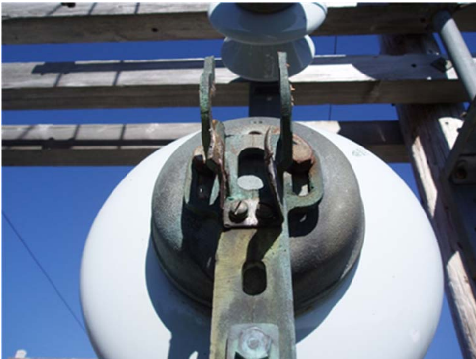
Figure 4: Misaligned blade terminal on 69 kV disconnect switch in Holyrood
