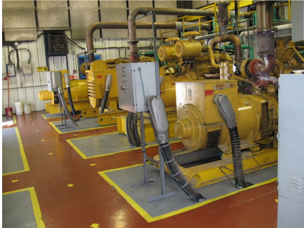
Figure 3: Cartwright Diesel Generators in Powerhouse
