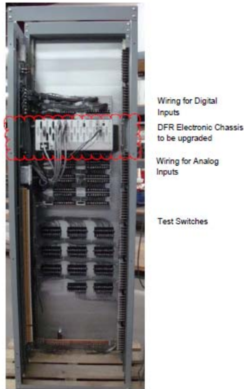
Figure 2: Mehta Tech DFR Cabinet Layout – Rear View
