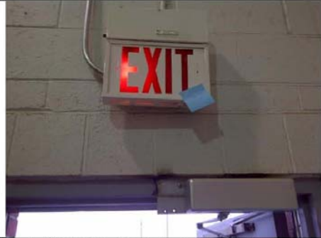
Photo #28: Exit Light with Faulty Test Switch
