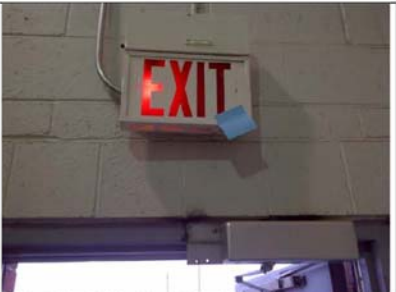
Photo #28: Exit Light with Faulty Test Switch
