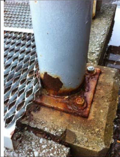
Photo #15: Ground Connection on Stair
