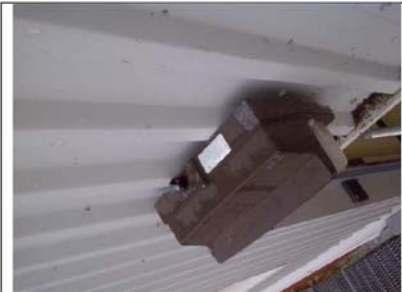
Photo #27: Wall Pack
