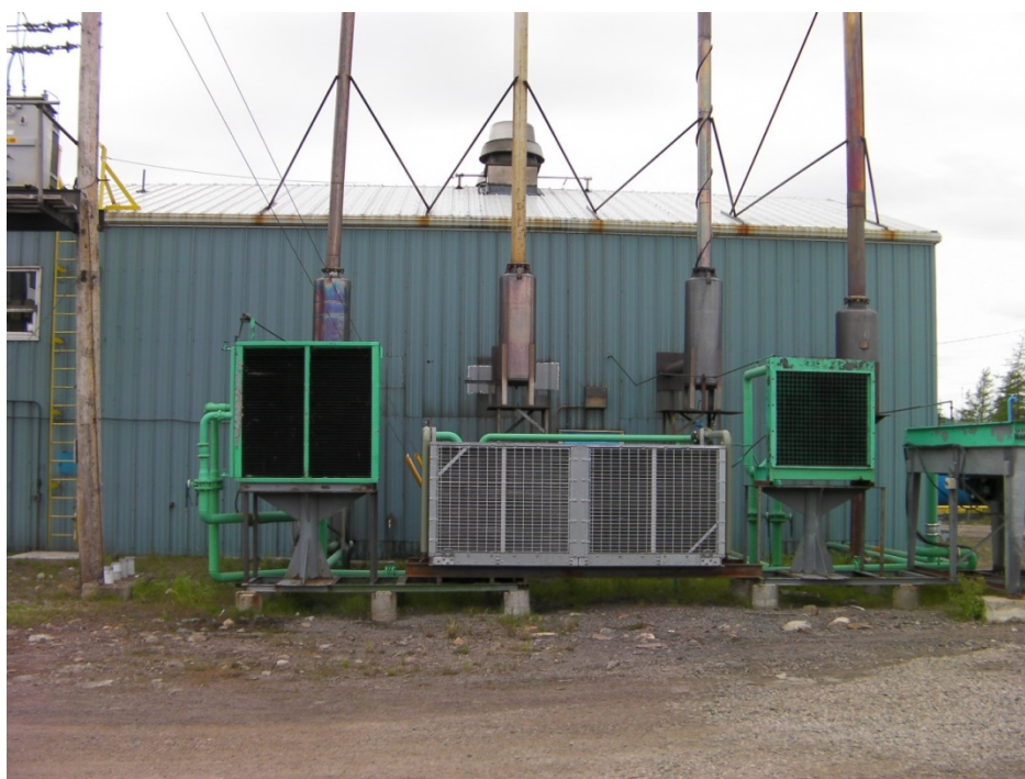
Figure 2: Cartwright – Diesel Generating Plant.
