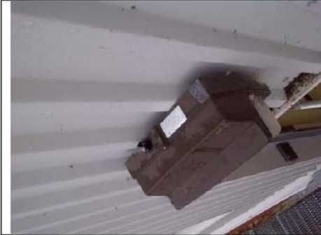
Photo #27: Wall Pack
