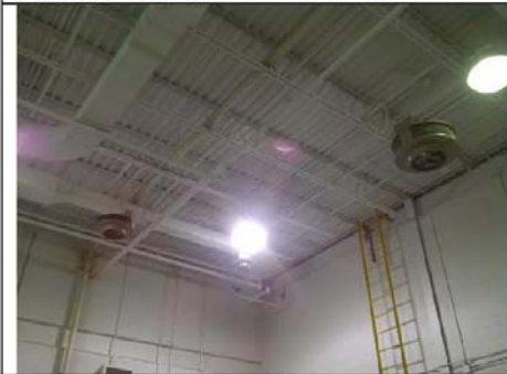
Photo #29: Metal Halide High Bays
