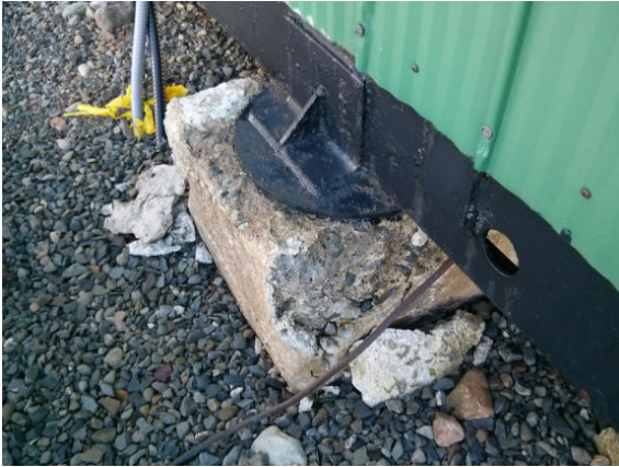
Figure 2: Cracked Concrete Foundation
