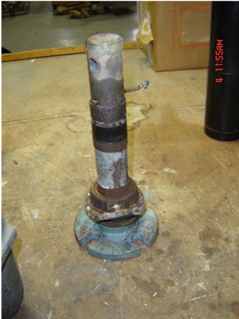
Figure 2: Broken Gear Drive from 230 kV disconnect switch in Holyrood
