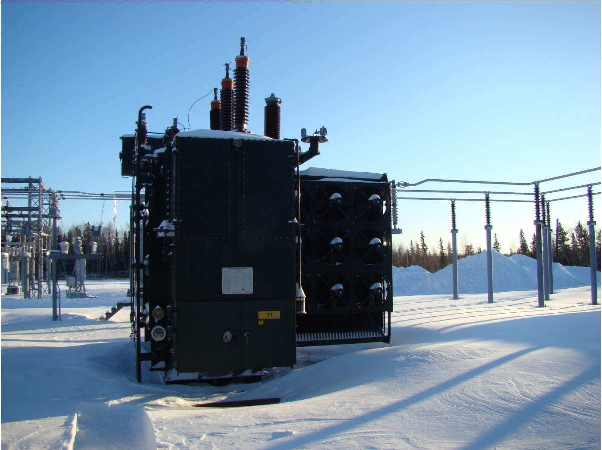
Figure 2: Spare 15/20/25 MVA Transformer (Happy Valley)
