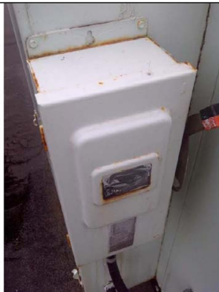
Photo #26: Rusting Disconnect
