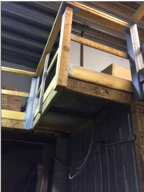
Photo 3: Mezzanine is structurally unsafe
