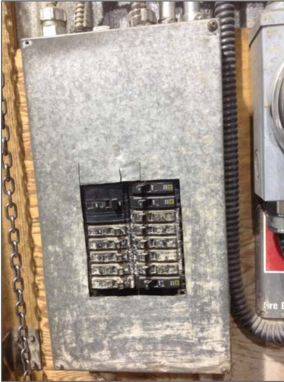
Photo 1: New panelboard required
