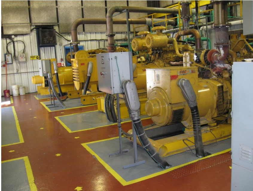
Figure 4: Cartwright - Diesel Generators in Powerhouse.
