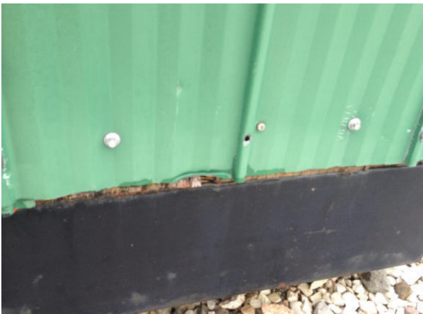
Figure 4: Exposed and Damaged Sheeting
