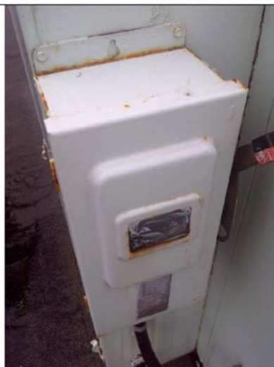
Photo #26: Rusting Disconnect
