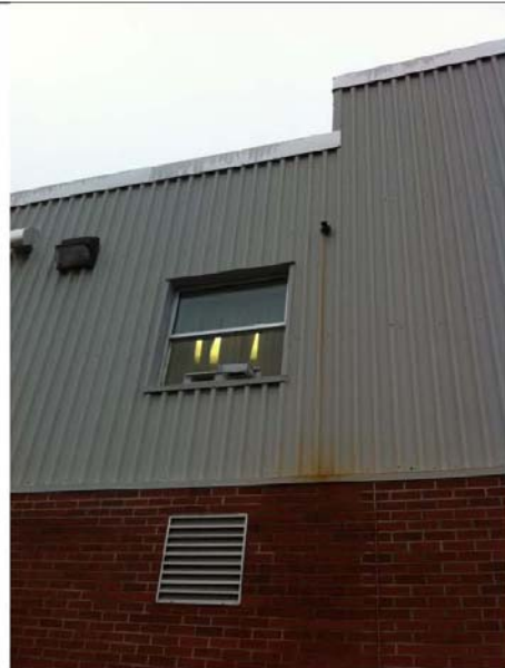
Photo #8: Rusting from Leaking test head
