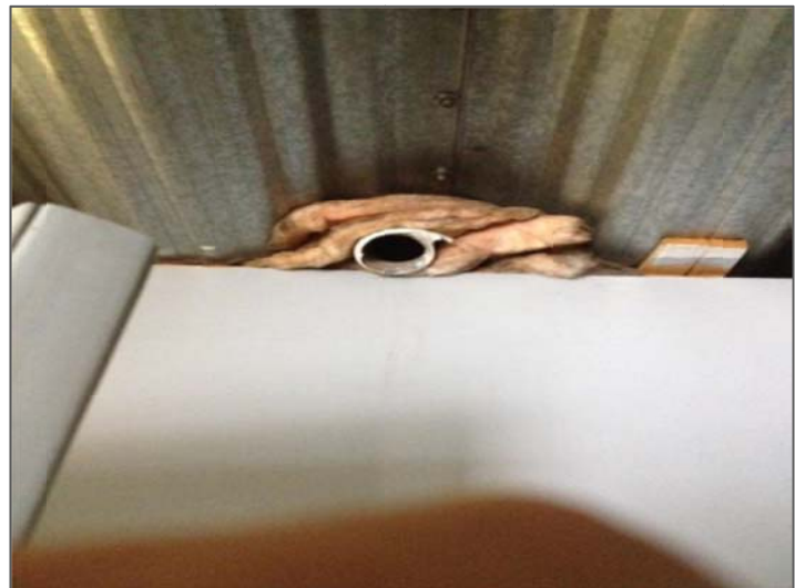
Photo 4: Washroom exhaust fan to be properly ducted to outdoors
