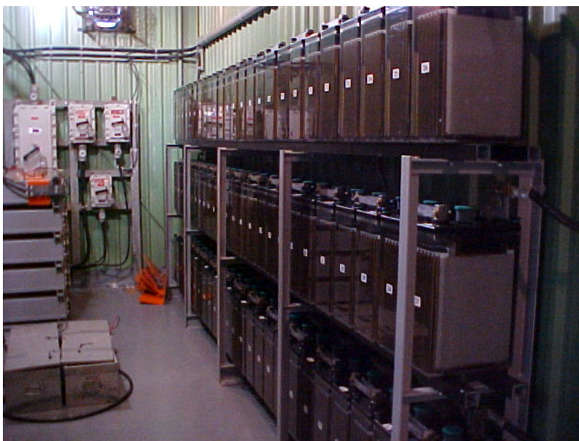
Figure 1: Flooded-cell battery (Stephenville)
