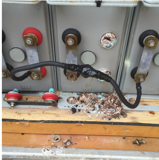
Figure 4: Failed VRLA Battery at Site #2
