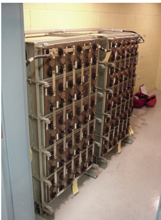
Figure 2: VRLA battery (Hinds Lake)
