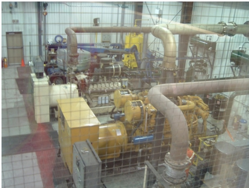
Figure 3: Nain – Diesel Generators in Powerhouse.
