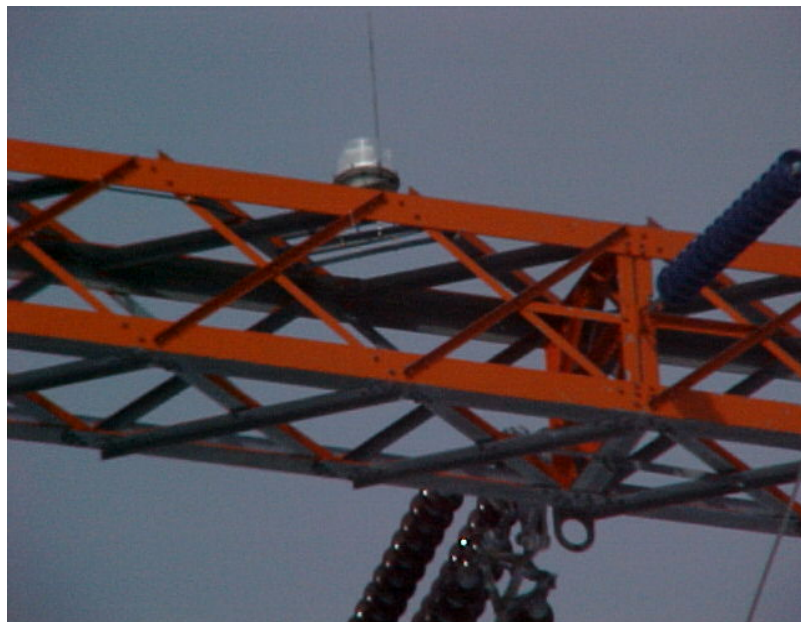
Figure 3: Flash Head on the 230kV structure
