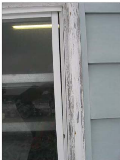
Figure 1: Window has Separated from Frame
