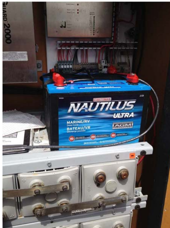
Figure 12 - Site 4 Replacement Batteries
