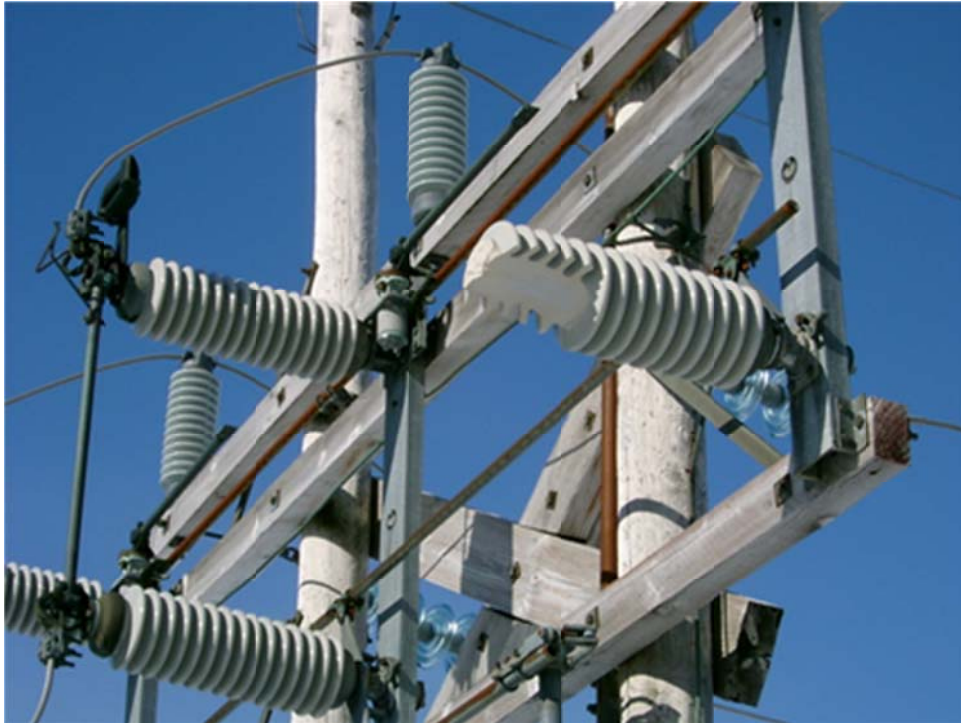
Figure 3: Broken insulator on 69 kV disconnect switch in Barchoix
