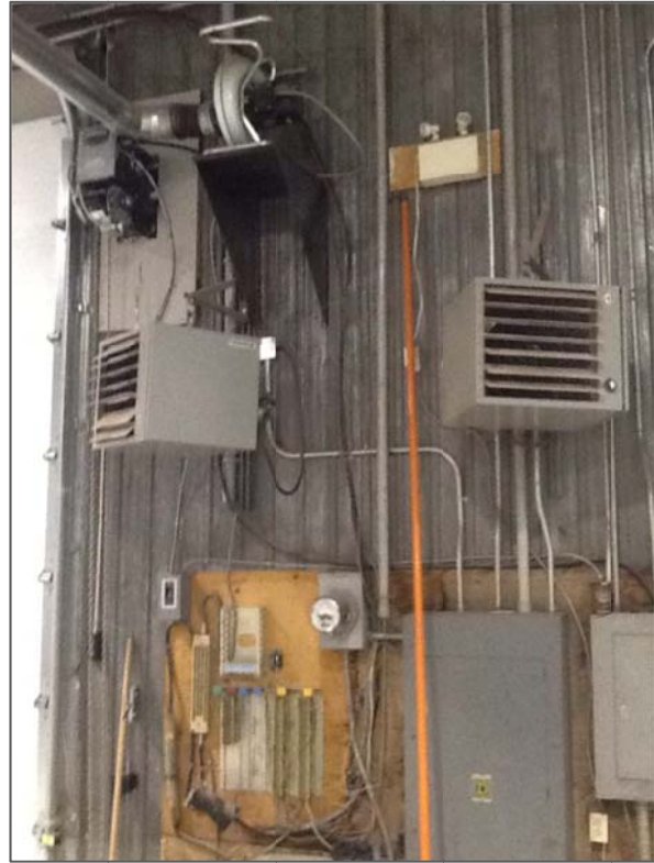
Photo 2: Welding shop heaters in poor condition
