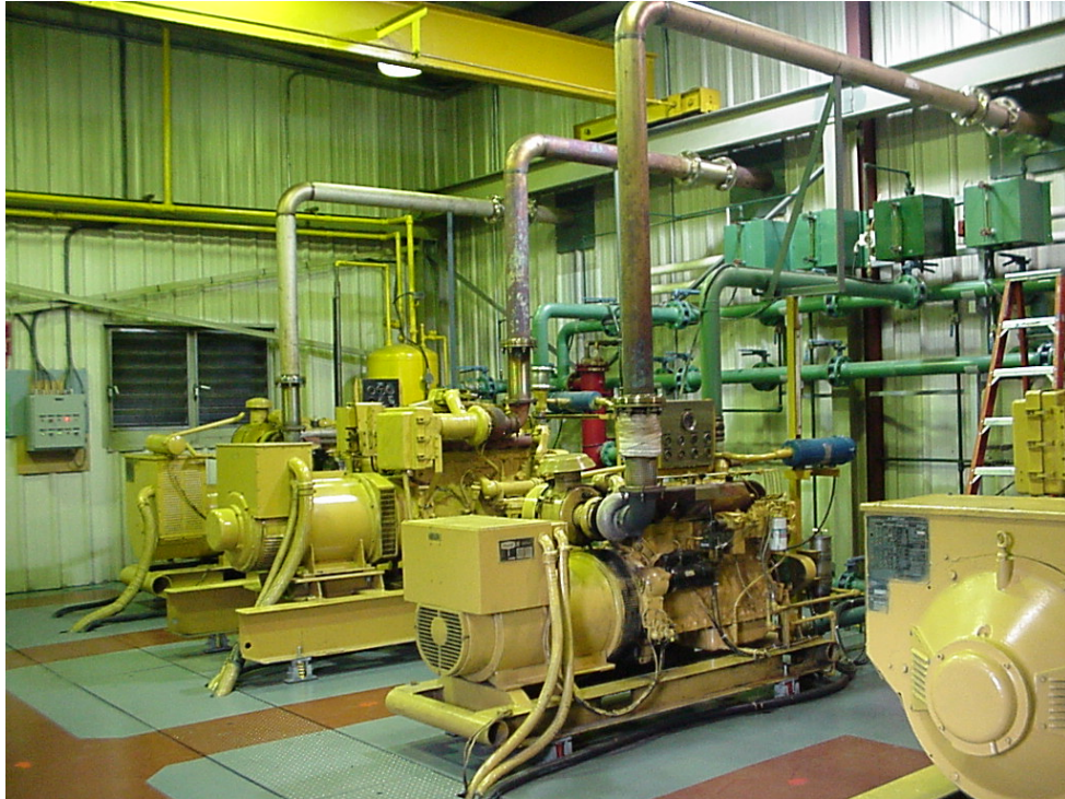
Figure 5: Charlottetown Diesel Generators in Powerhouse
