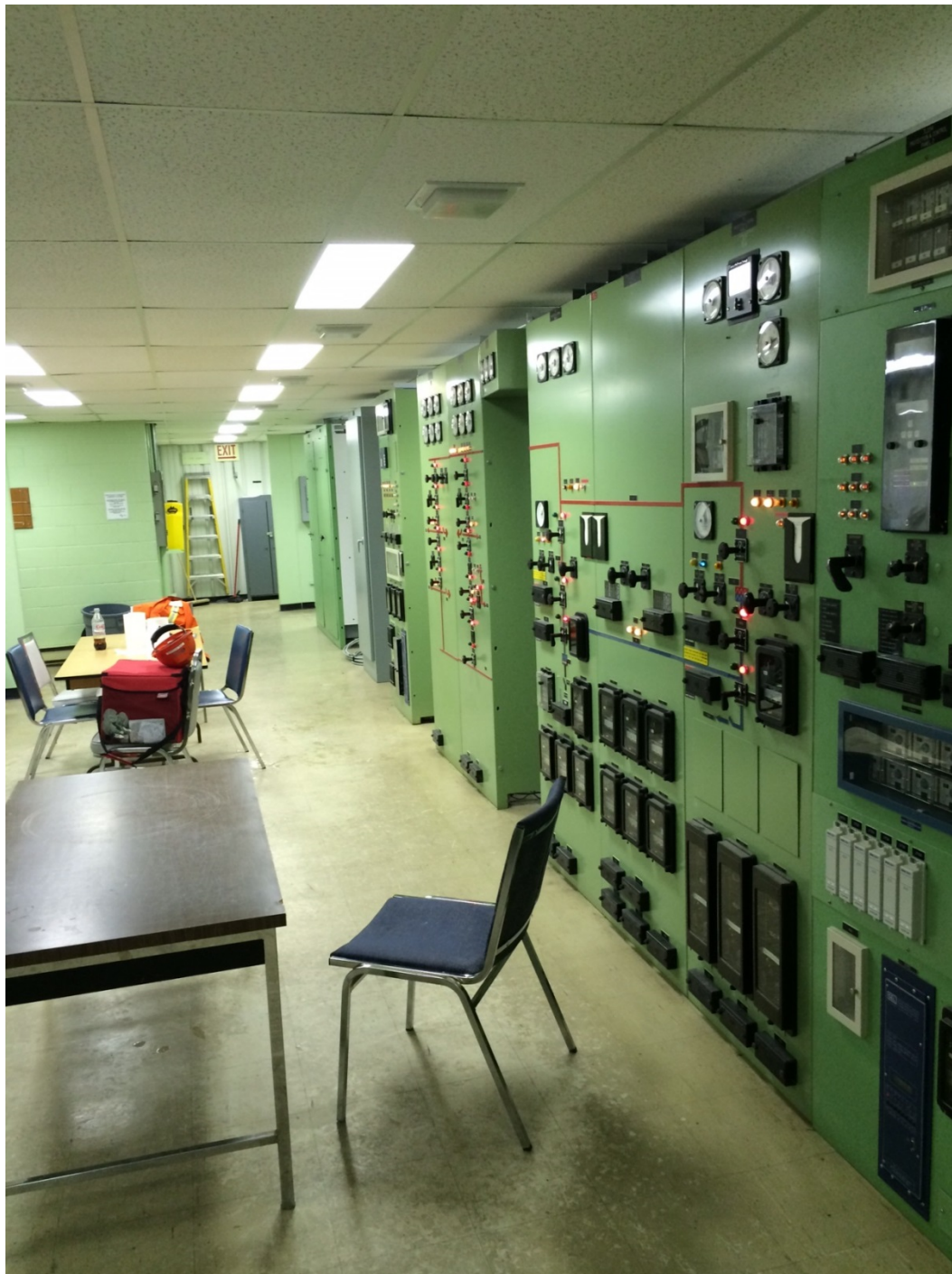
Figure 1: Bay d'Espoir Terminal Station – Control Panels and Cable Trays
