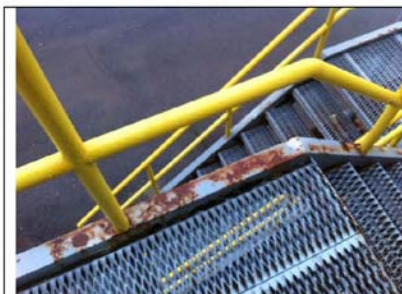
Photo #13: Rusting Stair Stringer
