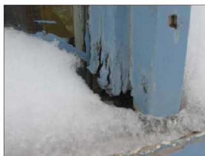
Figure 4: Rotten Sill and Siding – Storage Building
