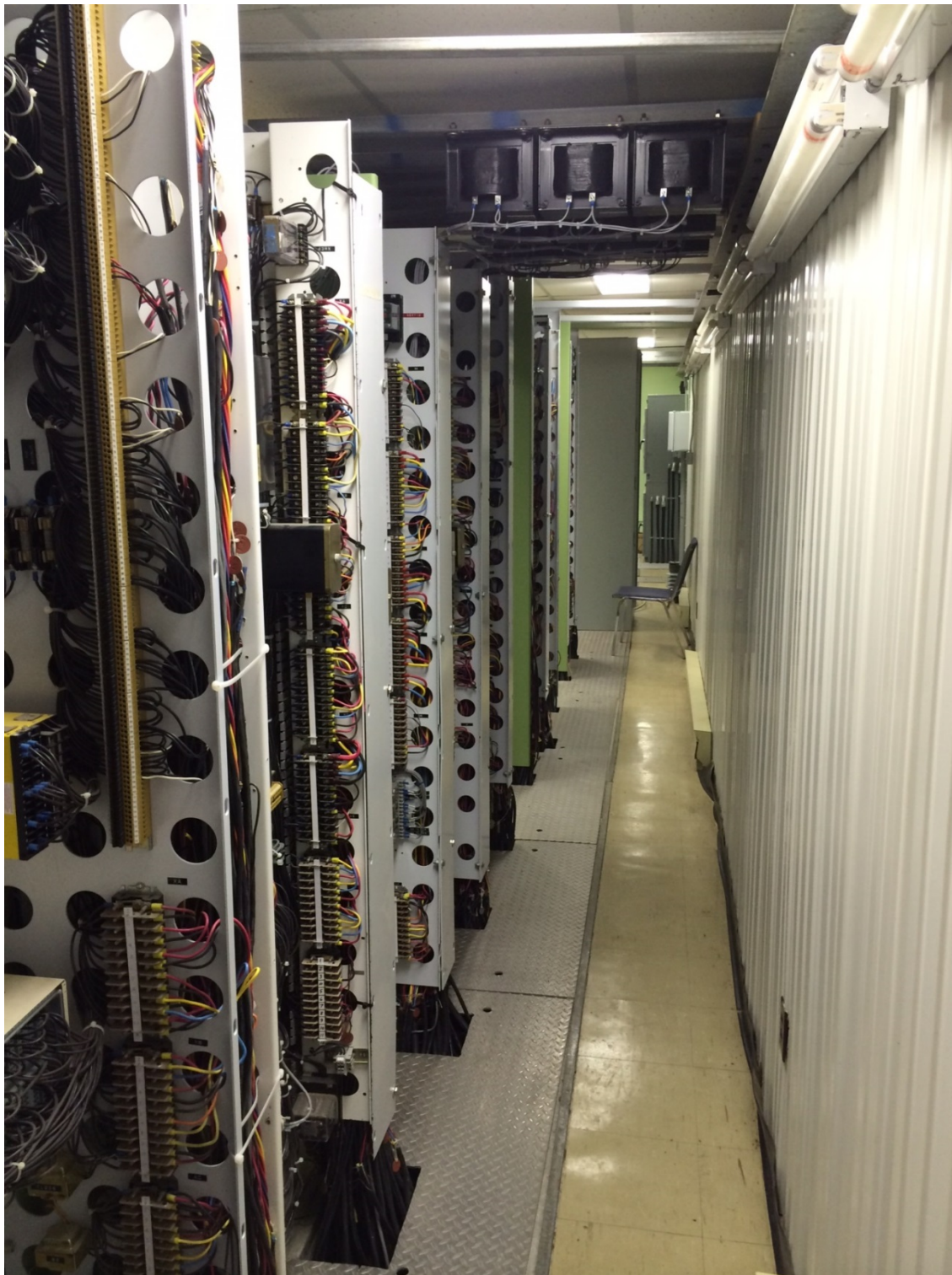
Figure 2: Bay d'Espoir Terminal Station – Inside Control Panels and Cable Trench
