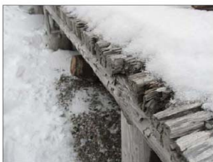
Figure 3: Rotten Storage Ramp Deck
