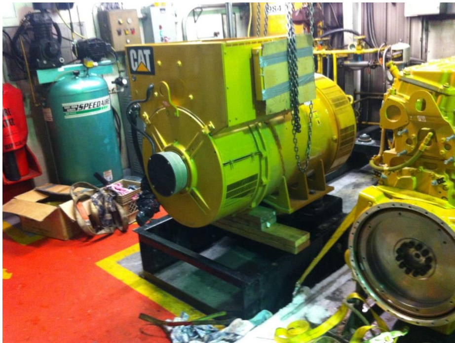
Photo 2: The New Generator (Left) and the New Engine (Right) Inside the Rigolet Plant
