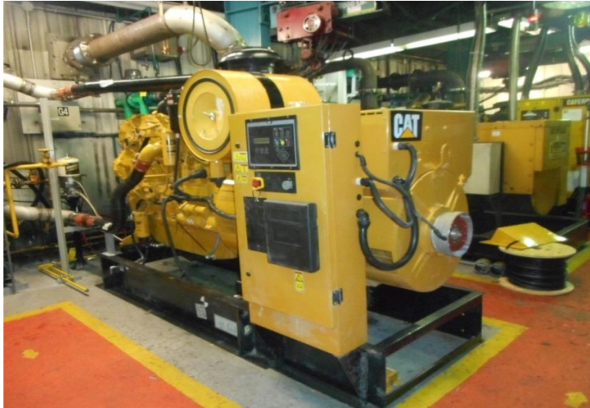
Figure 1: Unit 2101 Installed in place of Unit 2051
