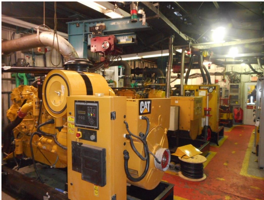
Photo 4: Unit 2101 Installed (Nearest Unit)
