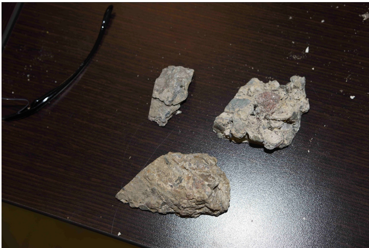
Photo 9: Stack No. 2 Small Pieces of Concrete Found on Lower Platform
