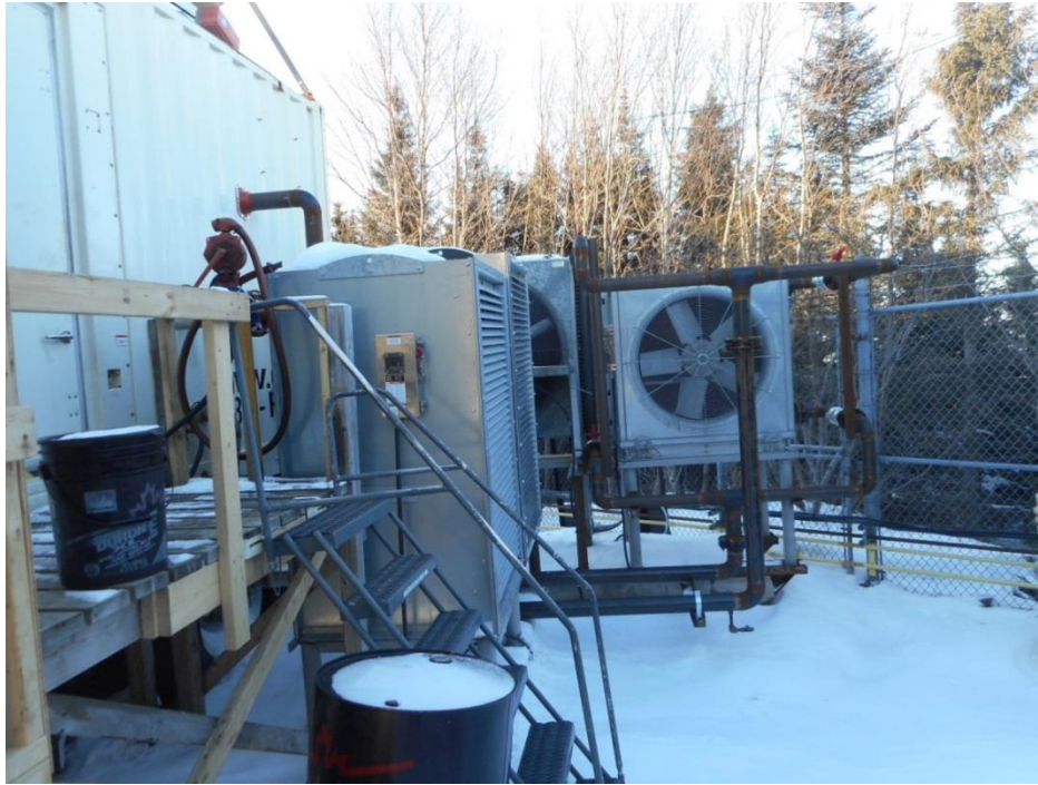
Photo 11: Unit 2088 Remote Cooling Equipment and Fuel Lines
