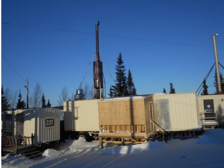
Figure 4: Winterized Units 2088 and 2089 and Newly Installed Unit 2102
