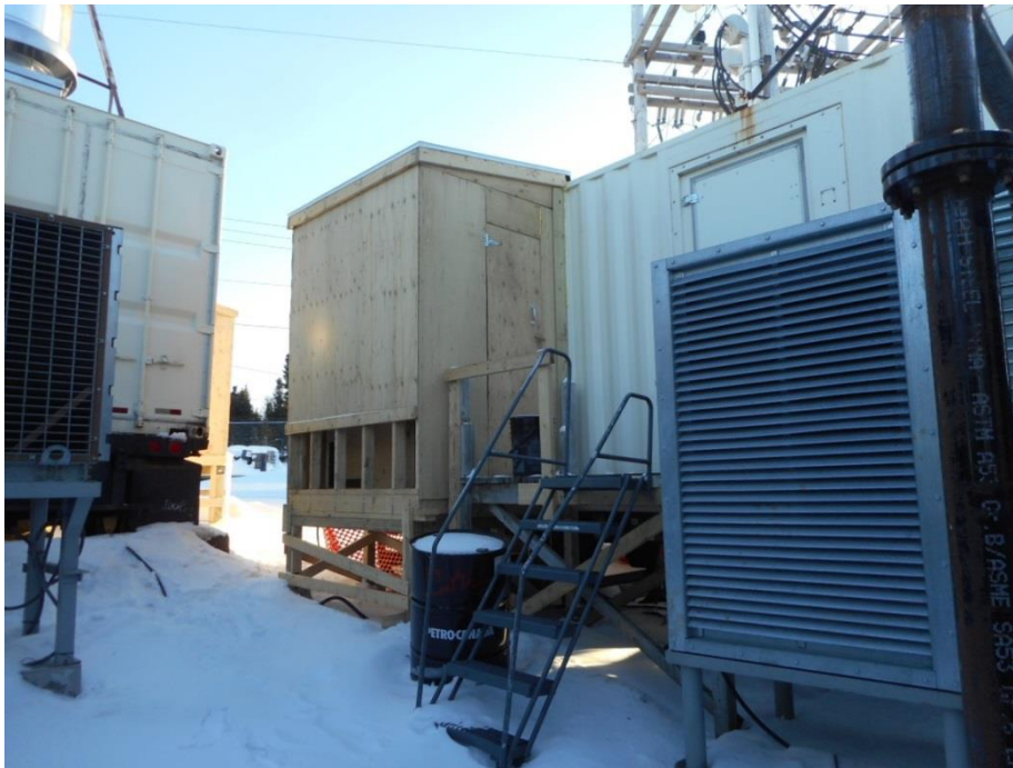
Photo 8: Unit 2088 Vestibule and Remote Cooling Equipment
