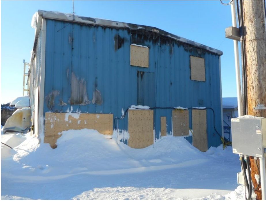
Photo 1: Charlottetown Diesel Generating Station Post Fire – Building Secured
