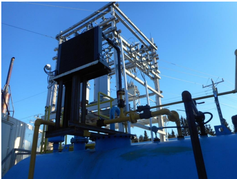
Photo 4: Substation and Fuel Supply System
