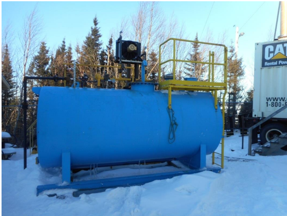
Photo 14: Intermediate Fuel Tank – Supply from Bulk Tanks to Mobile Units
