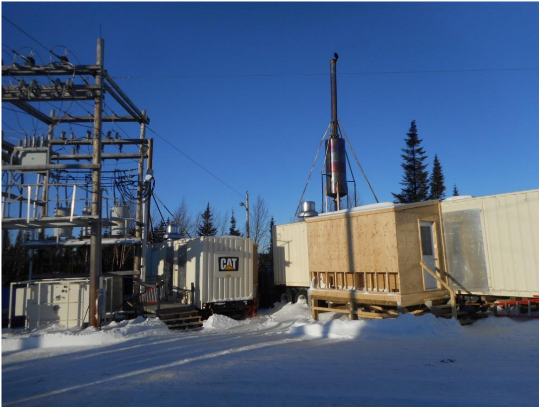
Figure 2: Substation and Winterized Gensets (Units 2088 and 2089)
