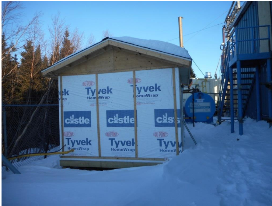
Photo 5: Equipment Enclosure for Fuel Pumps and Motor Starters
