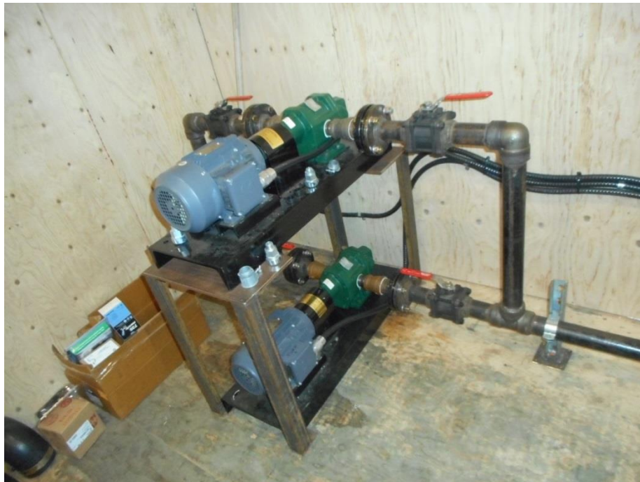
Photo 6: Fuel Transfer Pumps in Equipment Enclosure
