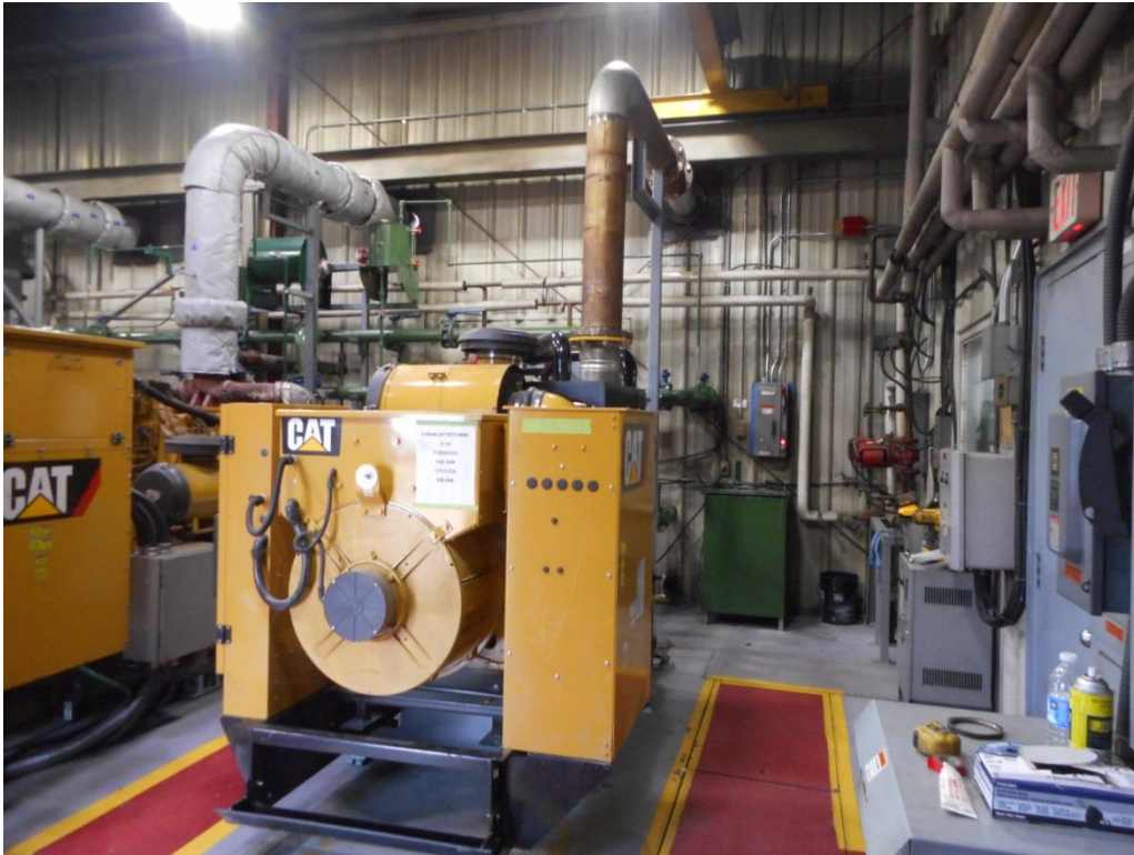
Figure 2: Charlottetown Diesel Generating Station Engine Hall (Before Fire) – Units 2092 and 2098
