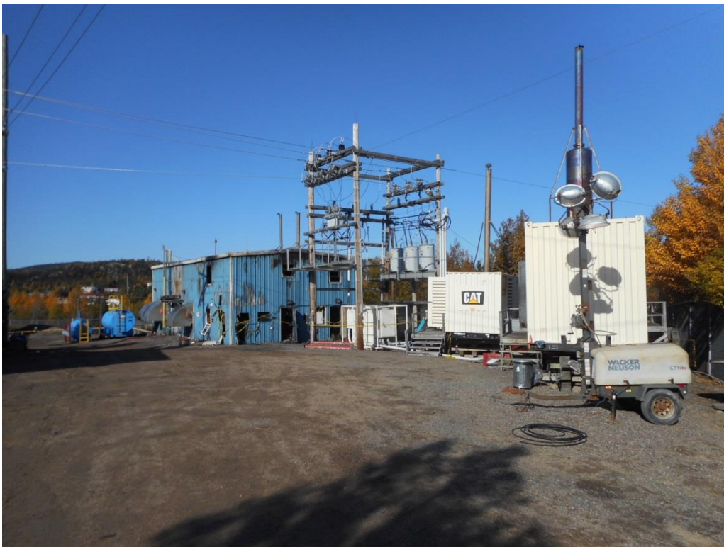
Figure 3: Mobile Gensets Immediately Following the Fire (No Winter Modifications)
