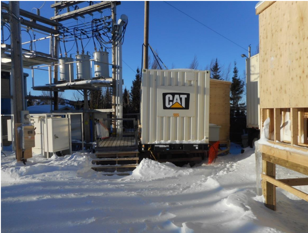
Photo 9: Unit 2088 and Substation
