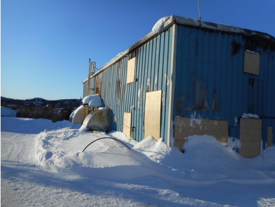
Photo 2: Charlottetown Diesel Generating Station Post Fire – Building Secured
