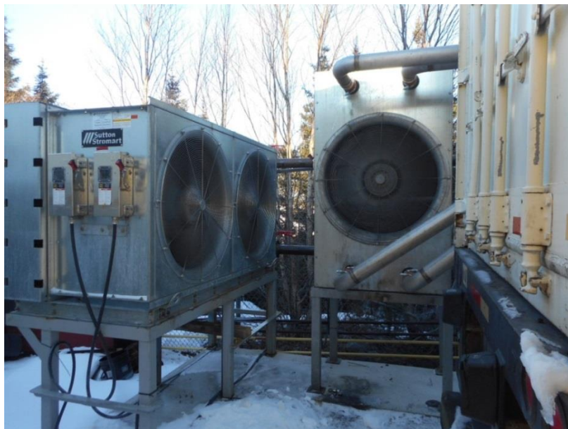
Photo 12: Unit 2089 Remote Cooling Equipment and Fuel Lines
