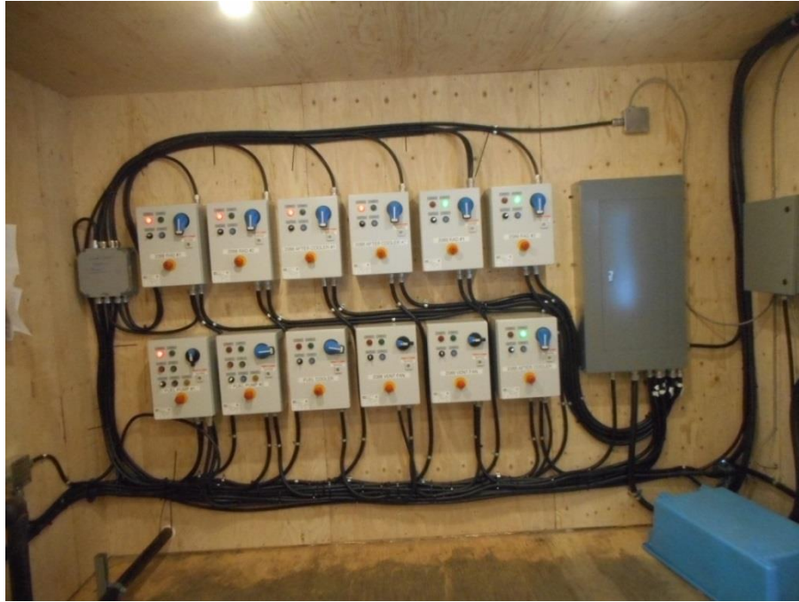
Photo 7: Motor Starters in Equipment Enclosure
