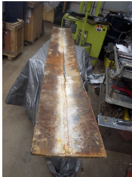
Figure 3-2: Penstock No. 1 - Failure occurred in 2017 (Ref. 3)
