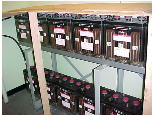
Figure 10: 125 Vdc Terminal Station Battery Bank
