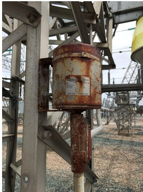
Figure 12: Corroded Ballast Requiring Replacement
