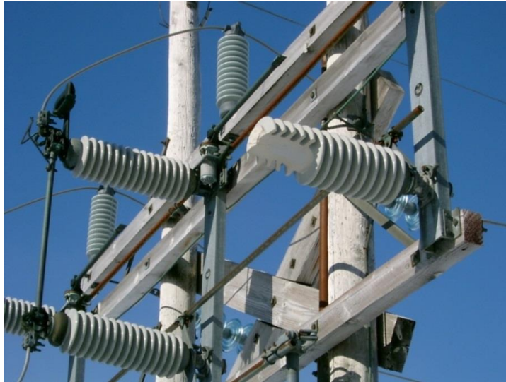
Figure 4: Broken Insulator on 69 kV Disconnect Switch
