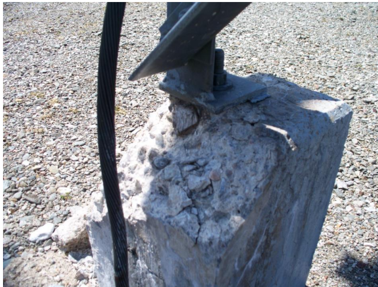
Figure 14: Structure B1T1 Bottom Brook Terminal Station
