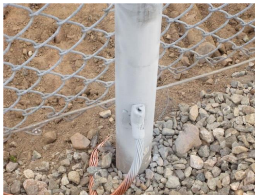
Figure 7: Typical Grounding Connection on Terminal Station Fence
