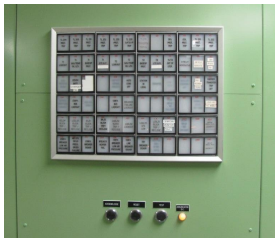
Figure 19: Annunciator Commonly Found in Hydro Terminal Stations
