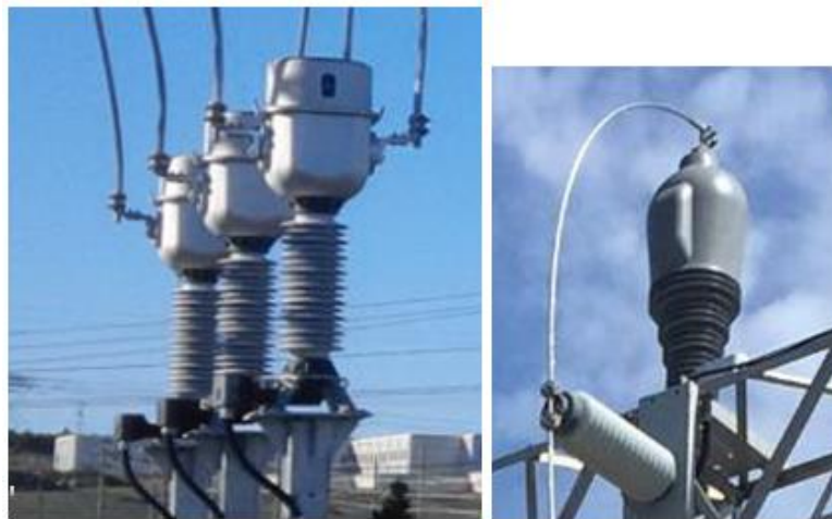
Figure 1: 69 kV CT (Left) and PT (Right)
