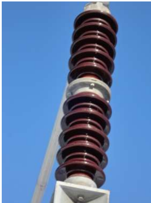
Figure 6: Multi-Cone Type Insulator Prone to Failure due to Cement Growth
