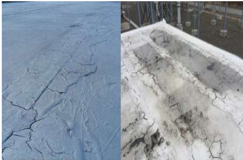
Figure 16: Terminal Station Control Buildings (Come by Chance and Sunnyside) Showing Cracking and Deterioration of the Roof Membrane System
