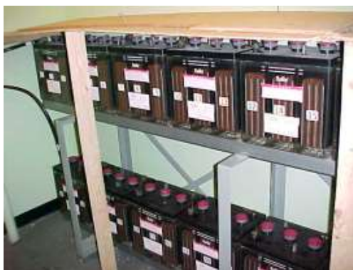
Figure 10: 125 Vdc Terminal Station Battery Bank
