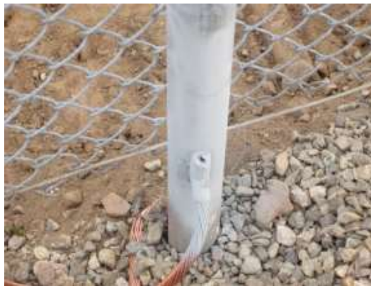
Figure 7: Typical Grounding Connection on Terminal Station Fence
