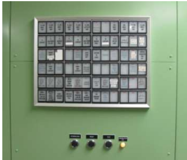
Figure 19: Annunciator Commonly Found in Hydro Terminal Stations
