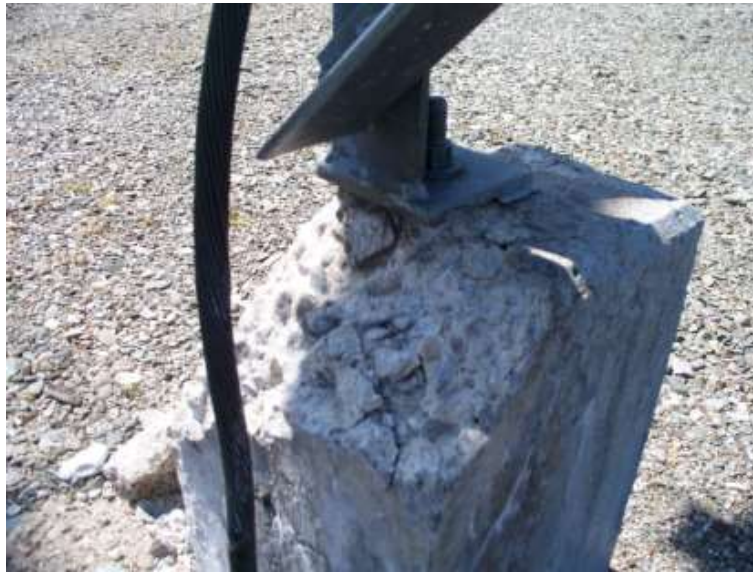
Figure 14: Structure B1T1 Bottom Brook Terminal Station
