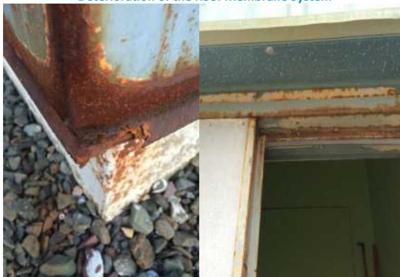
Figure 17: Building Exterior Cladding and Exterior Doorways Displaying Severe Rusting and Deterioration
