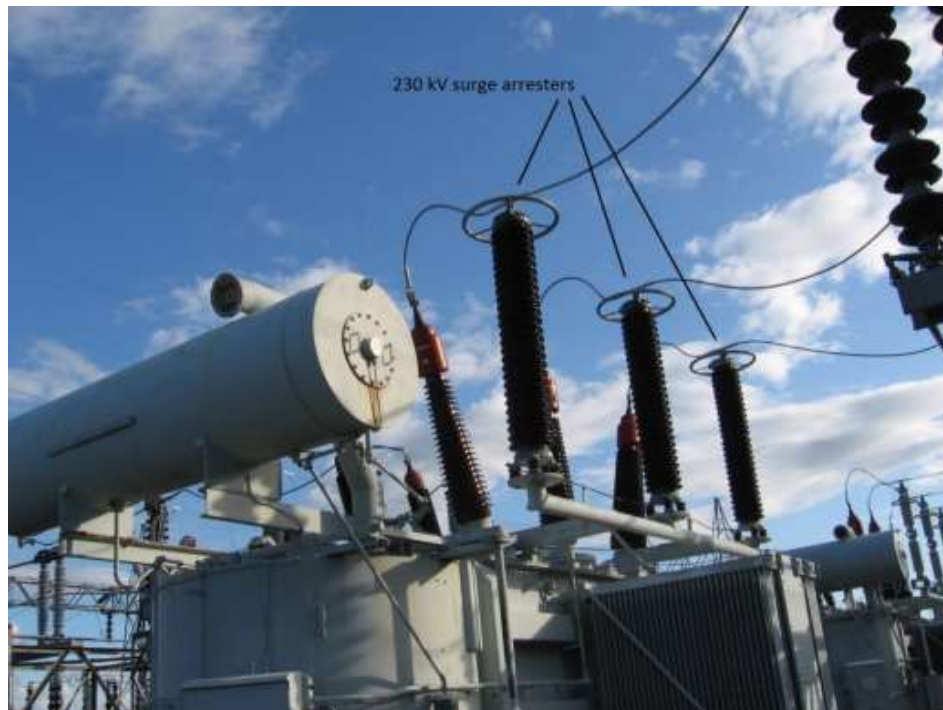
Figure 5: Western Avalon Terminal Station Transformer T3 230 kV Surge Arresters
