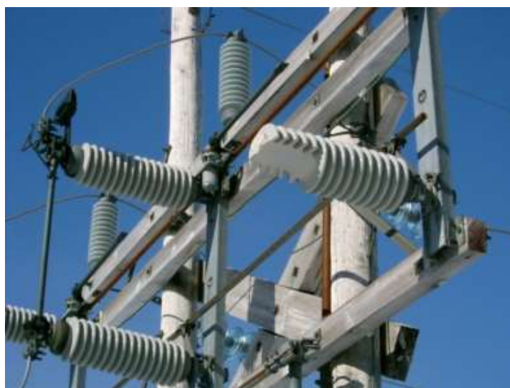
Figure 4: Broken Insulator on 69 kV Disconnect Switch
