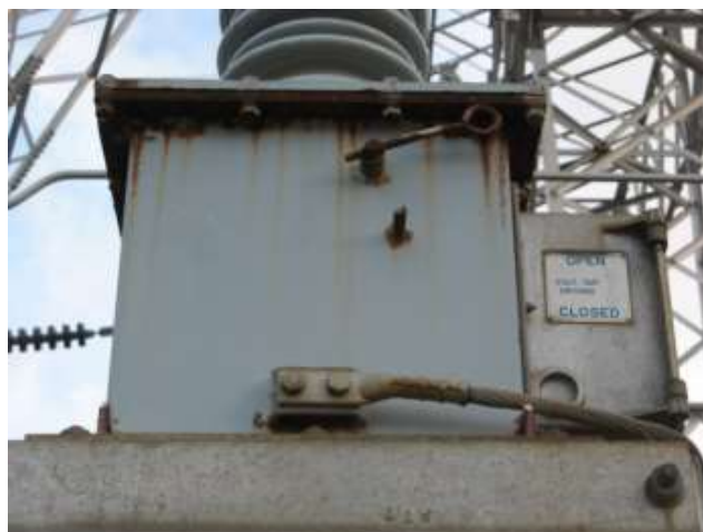
Figure 2: Rusting Potential Transformer
