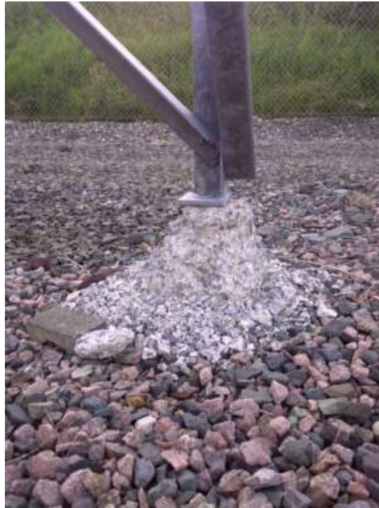
Figure 15: Structure L01L37-1 Western Avalon Terminal Station
