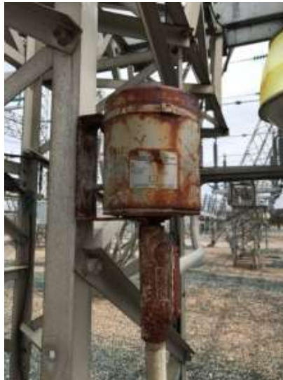
Figure 12: Corroded Ballast Requiring Replacement
