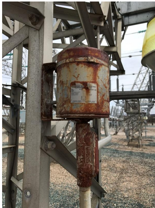
Figure 12: Corroded Ballast Requiring Replacement
