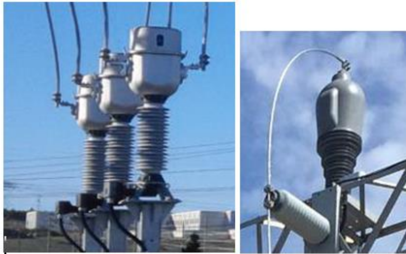
Figure 1: 69 kV CT (Left) and PT (Right)
