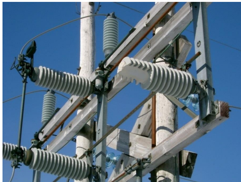
Figure 4: Broken Insulator on 69 kV Disconnect Switch
