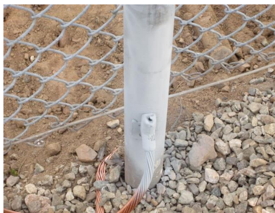
Figure 7: Typical Grounding Connection on Terminal Station Fence
