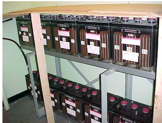
Figure 10: 125 Vdc Terminal Station Battery Bank
